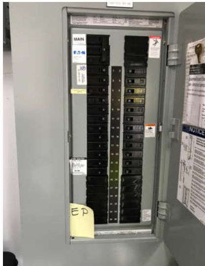
B.O.H. ELECTRICAL PANEL UPPER LEVEL
