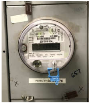
TERMINAL 1 CONCOURSE B ELECTRICAL METER
